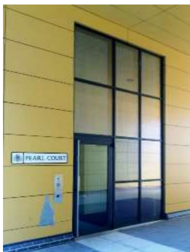
STS202 BR2 Tested Mild Steel Doorset within Curtain Walling Facade
